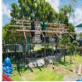
Construction of a new ram pump testing shed is underway-was completed that same month
