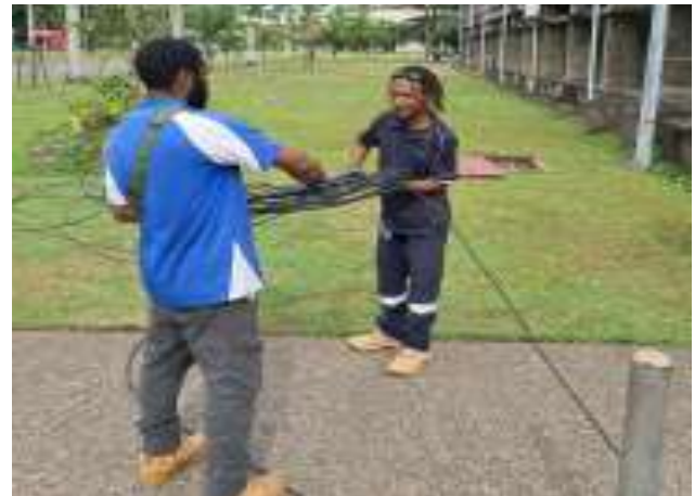
10Gbps Fibre-optic Cabling
